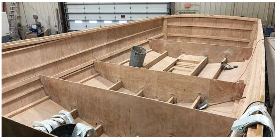
Weaver's conventional wood/epoxy composite construction method includes Douglas-fir stringers and stiffeners, Okoume plywood planking and bulkheads, and fiberglass sheathing inside and out on hull, deck, and cabin structures.
