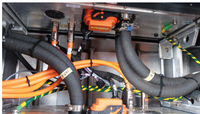
Top —Heron’s ample and protected pilothouse provides good sight lines over the forward work deck. Above —A hatch in the pilothouse sole grants access to electrical connections and cooling inputs for the boat’s two 800V batteries.
