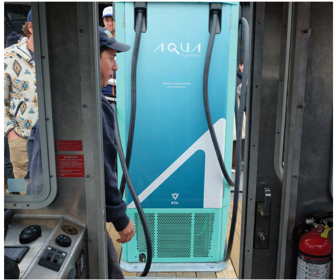
Willy Leathers pulls Heron up to the new level -3, 75 kWh dockside charger at the Gulf of Maine Research Institute's Wright's Wharf facility in Portland, Maine.
