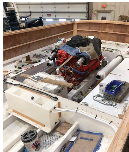
The single 900-hp Scania DI 16 diesel rests on its engine beds as systems and structure are built in around it.
