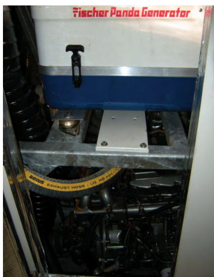
All too often a generator is stuffed into too small a space with very poor access for maintenance. This generator also inhibits access to the propulsion engine located below it.
