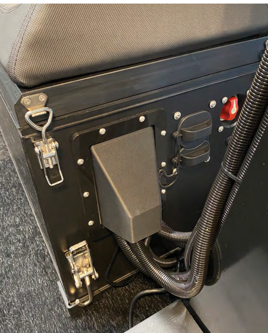
The tidy battery box and console installations are possible in part because all connections for steering and throttle control are electrical, not mechanical.
