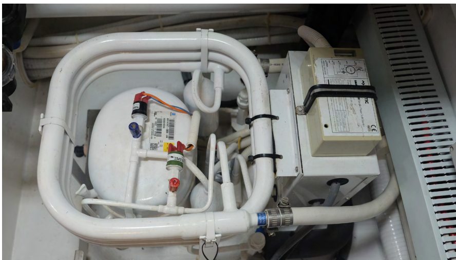
High-draw appliances like this air conditioner commonly exceed the capacity of alternators and require a generator.
