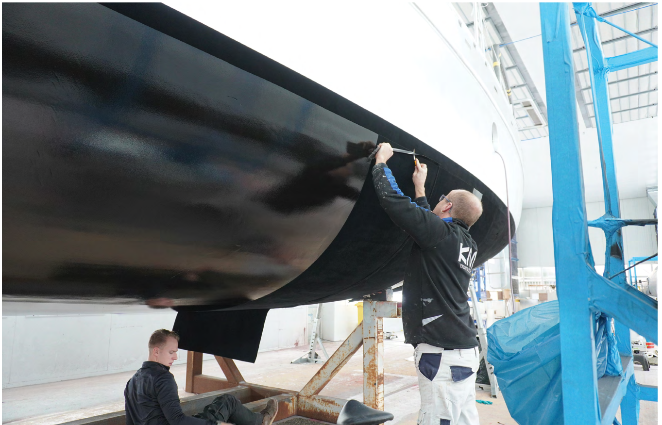
Many of the 900 boats fitted with Finsulate are recreational sailing vessels, for which the material is well suited. Installation is similar to hanging wallpaper.
