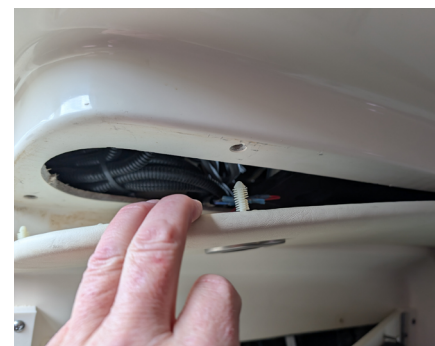
This removable panel is better than no access, but the wiring behind it is still crammed in, leaving little workable room.
