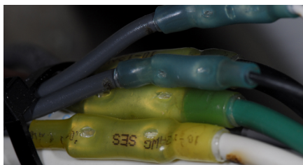
Wire unions should be properly sealed with heat-shrink crimped connectors to protect them from moisture. These have been compromised by incorrect crimping.
